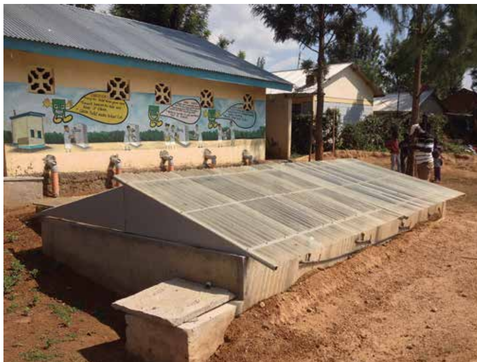
Biogas digester in Nyabirongo girls school, Migori Region, Kenya
